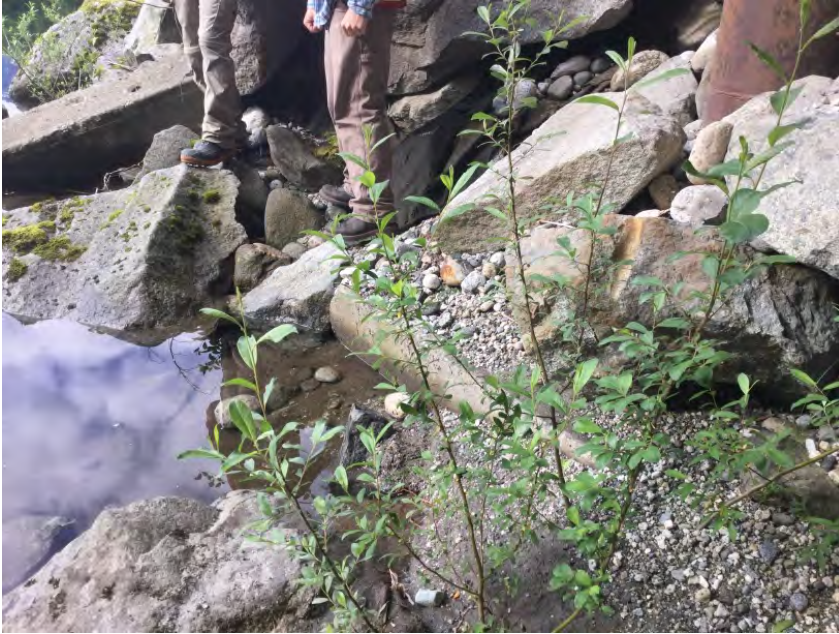
Downstream right footing exposed
