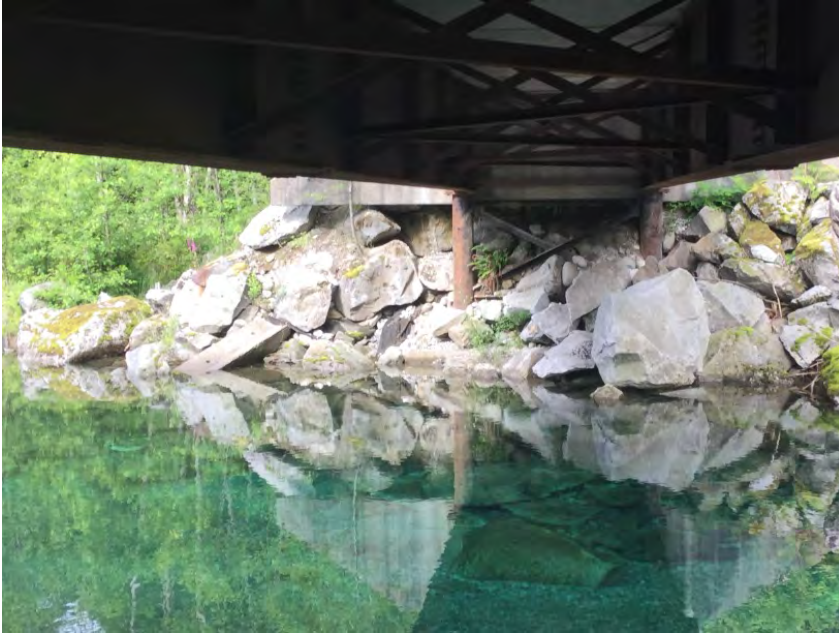
Downstream right bank riprap scour
