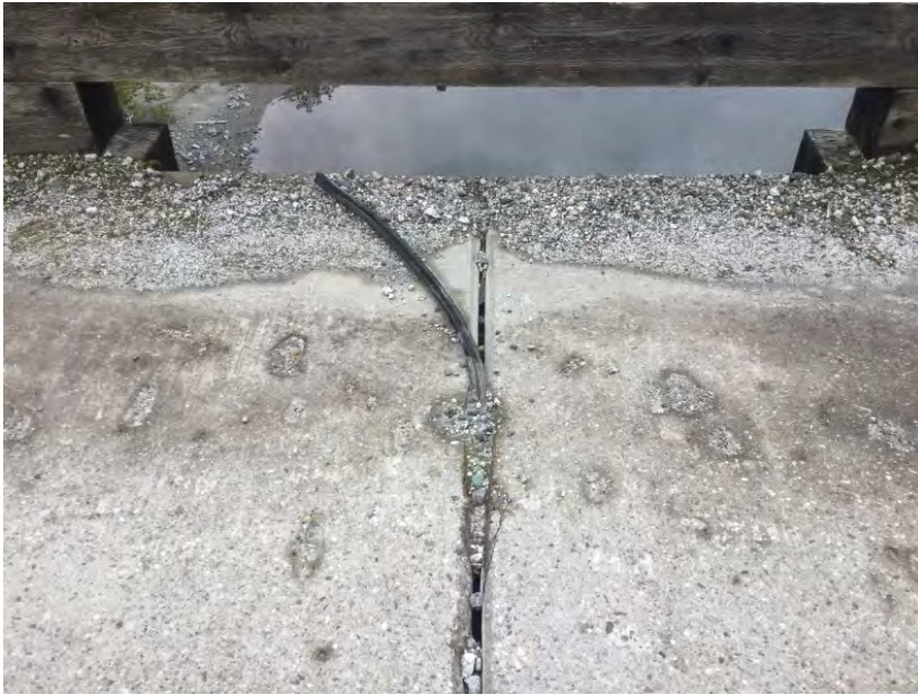
Seals between deck panels failing throughout
