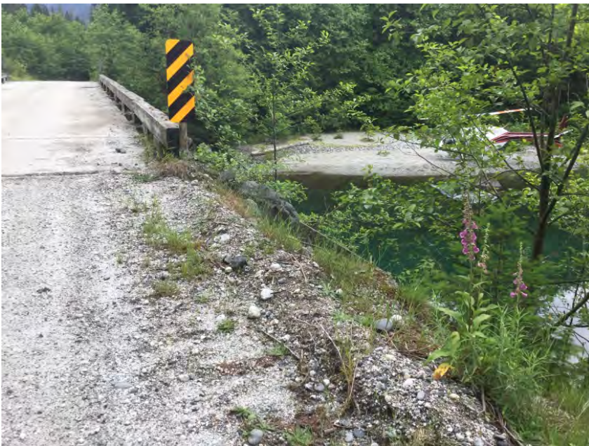
Missing no post barriers
