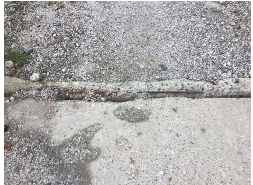
Right bank ballast wall damage
